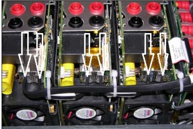
Figure 186 Communication Cable Connections
